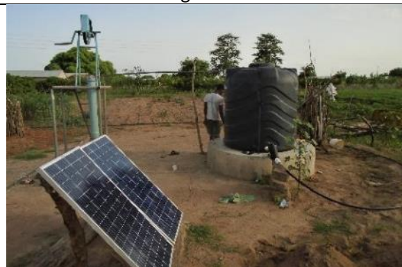
1 pump ZL 50-20N is replacing a Rope pump. It pumps into a tank and is used for drip irrigation.
