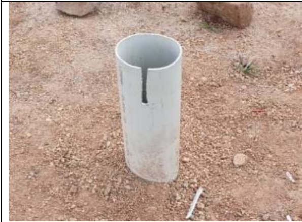
Slot in the casing to accommodate cabling in the well head.
